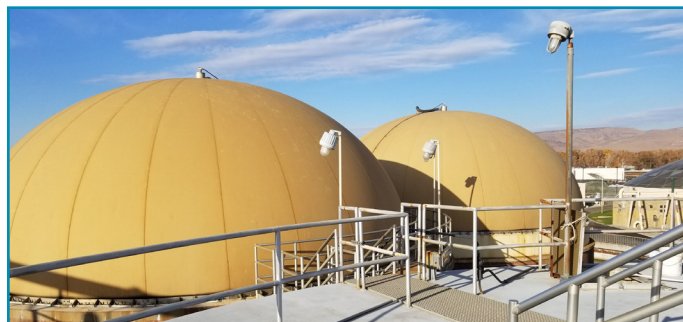
Typical membrane gas holder covers on secondary anaerobic digesters as installed at the City of Yakima.
