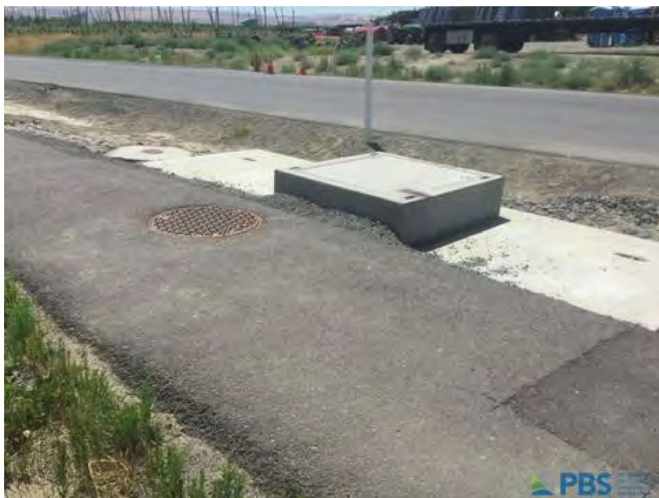
Photo 26. Utility access manholes.
