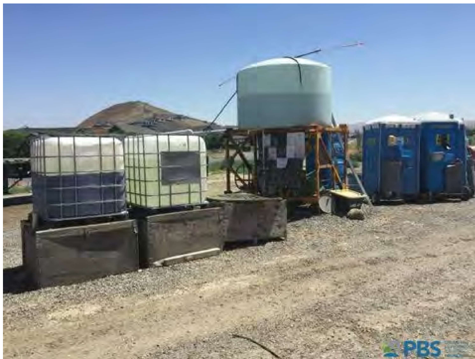
Photo 39. Lime sulfur tanks.
