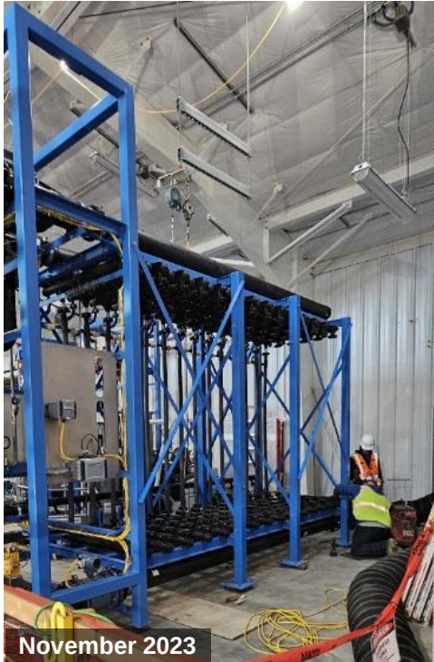
Filter rack installation in Central Plateau Water Treatment Facility
