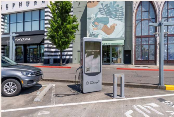
EV CHARGING STATION ADS
