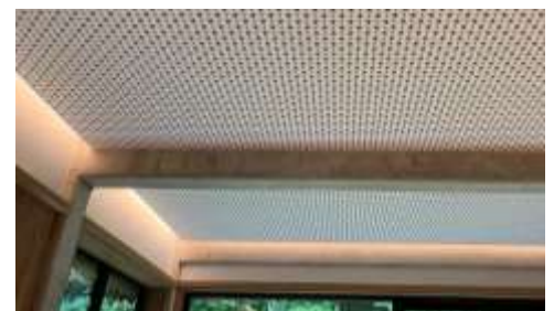
Ceiling installed acoustic panels in a common area. Photo courtesy of Schemata Workshop.
