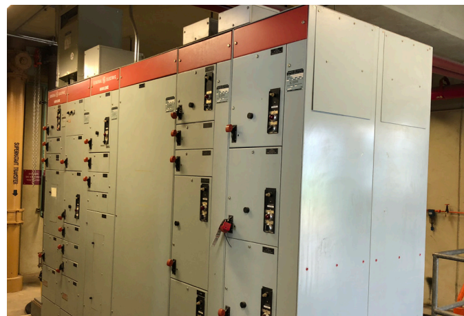
Existing MCC at the City of Richland 's WWTP Digester Facility
