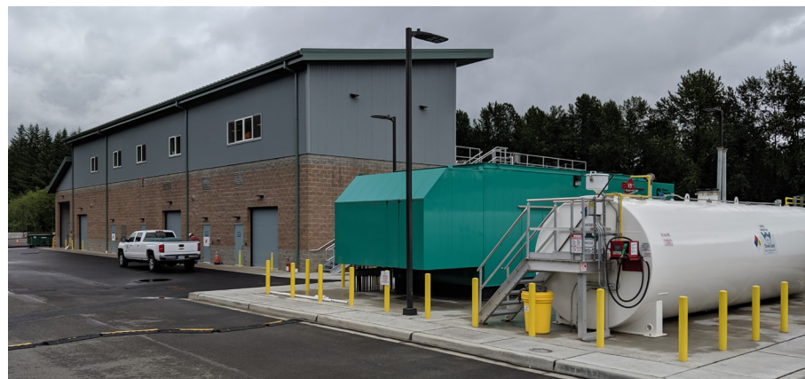
New 1,500 kW diesel standby generator at the WRF
