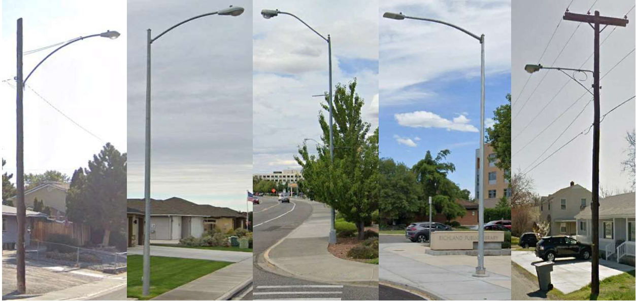
Figure 1. City of Richland Street Light Examples (Google Earth Street View Imagery, 2020)
