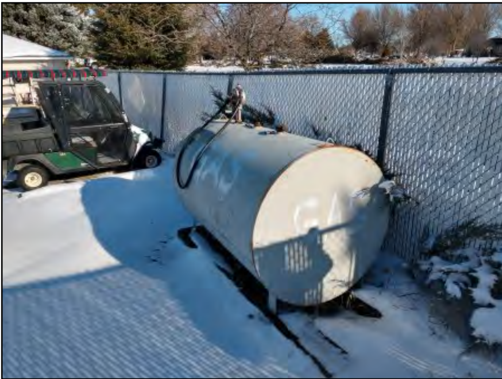
Gas AST at the site
