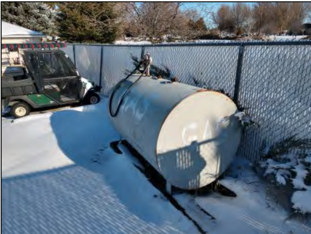
Gas AST at the site
